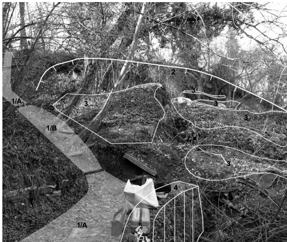
Photo 2. Main features of the investigated landslide (Photo by G. Varga). 1/A – former footpath, 1/B – destroyed stairs, 2 – head scarp, 3 – blocks of landslide, 4 – counterfort
