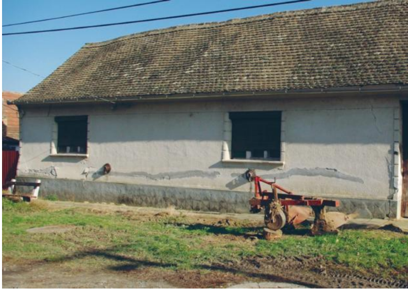
Photo 2. Damages to a residential property at the southern part of Dunaszekcső. Foundation and the walls of the house were ruptured due to shear stresses.
