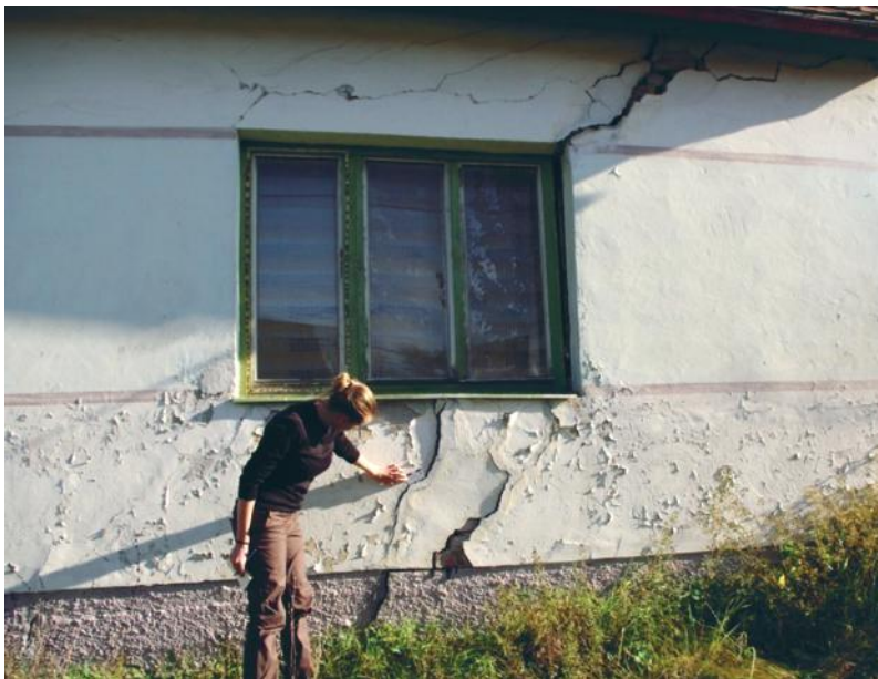
Photo 1. Building damage on an abandoned house at the southern part of Dunaszekcső. Foundation of the house was broken.
