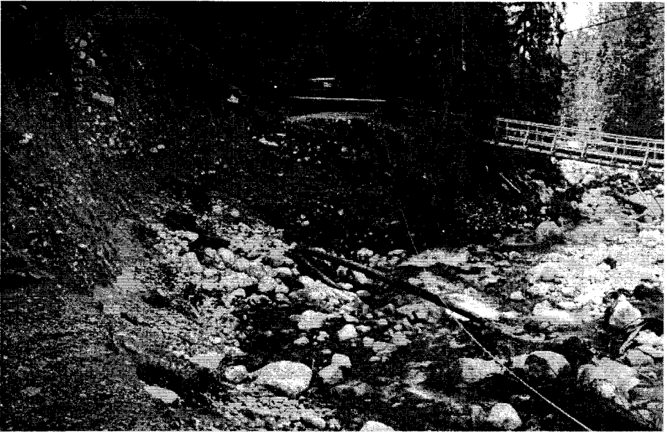
Photo 4. Erosion undercut 30 m long and 10 m wide within the main road from Brzeziny to Hala Gąsienicowa. The volume of eroded material is calculated to be around 1,200–1,400 cu. m
